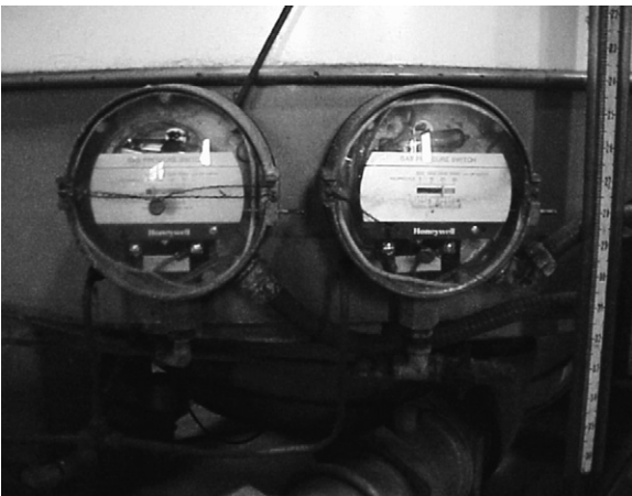
Exhibit 2. Typical high/low fuel pressure switches to verify fuel pressures are in the proper range.
