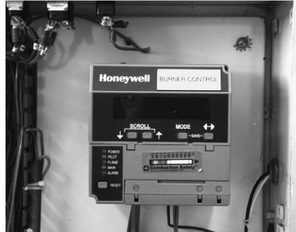
Exhibit 4. The BMS or burner management system is the brain that monitors/directs safe firing and operations.
